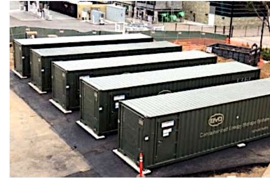
BYD Battery (2.5 MW/ 5 MWh)
